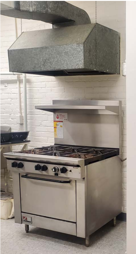
First floor, Gas cook stove & hood
