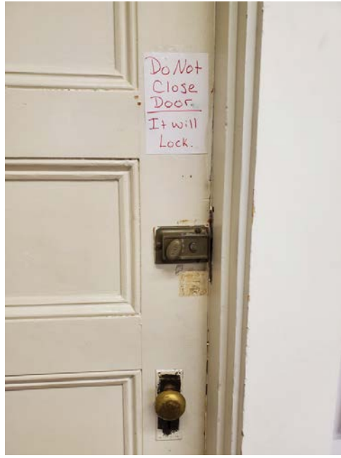
Non-compliant Door Hardware
