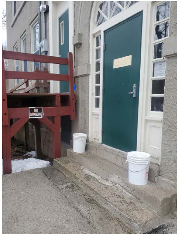
East side, entry door- failing concrete stairs
