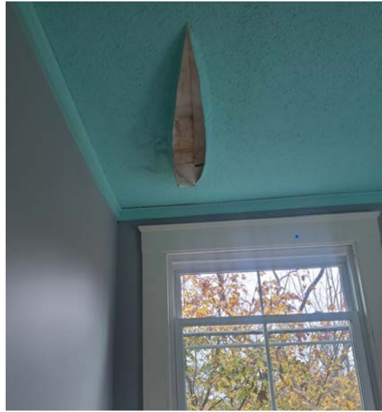
Third floor, ceiling damage
